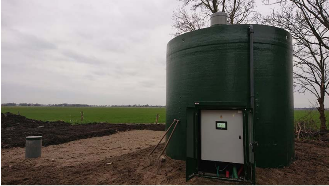
Figure 3, BEVER treatment system in operation
